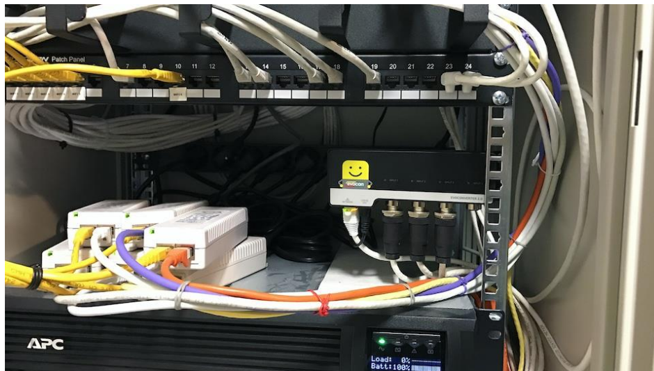
Evocon's implementation process consists of cabling the IIoT devices and sensors on the production line and establishing an internet connection.
